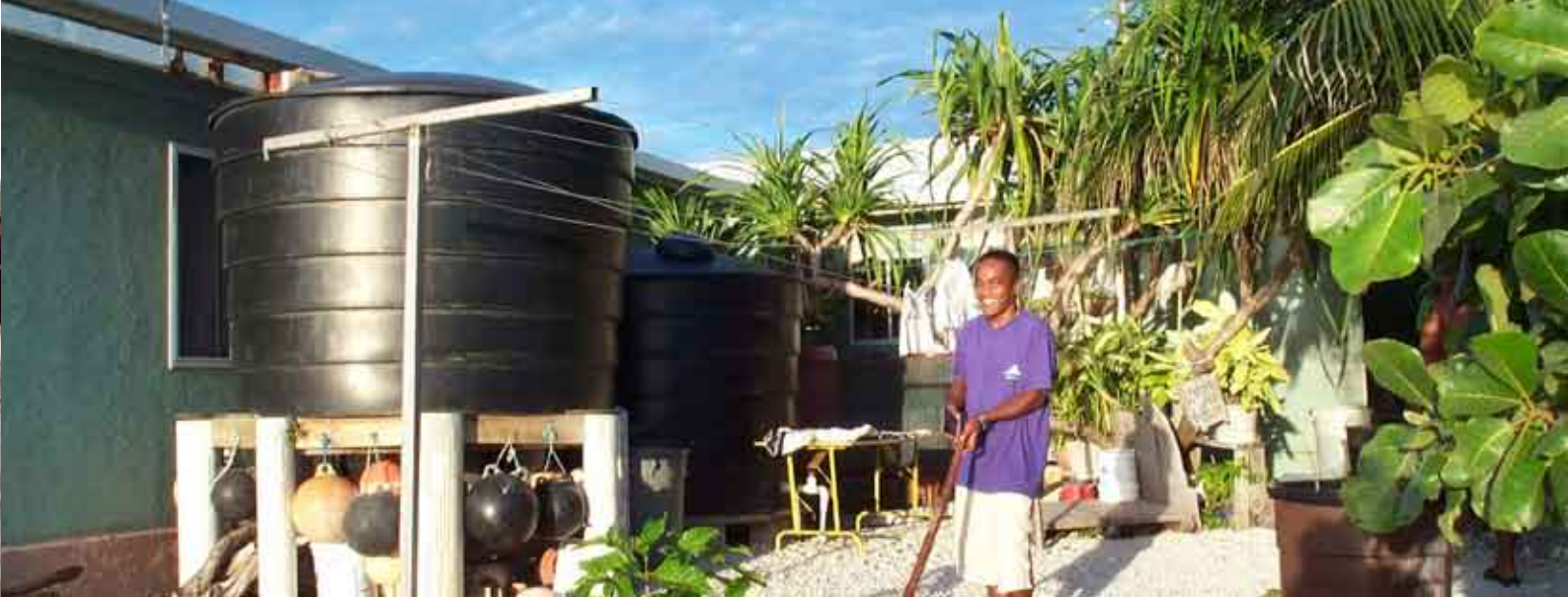
Water tanks on Majuro, Republic of Marshall Islands. ©SOPAC
