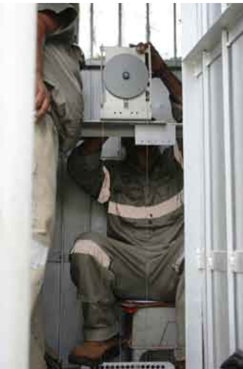
The new logger is installed.
